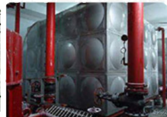
Fire and tank water level
